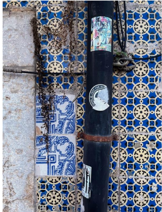
Figure 12 Building Façade (Graça), two tiles have been replaced by tiles with different pattern, author’s photograph (2022).
