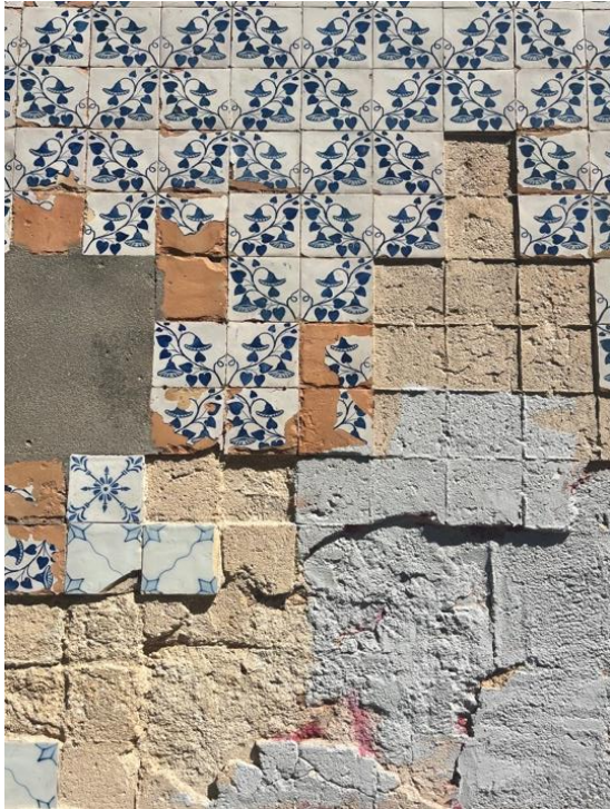
Figure 13 Building Façade (Mouraria), many tiles have fallen off, some have been replaced, author’s photograph (2023).
