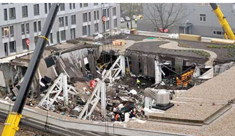
Faulty girder connections could have caused the collapse Copyright: Roman Koksarov
