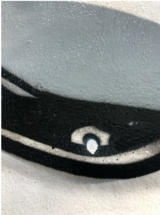
Fig. Att. 97 – Wetting detail in the application of the Pro-Art protective coating.
