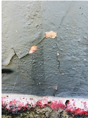
Fig. Att. 76 – Detail of detachment in an area with a repaint in the grey chromatic layer.
