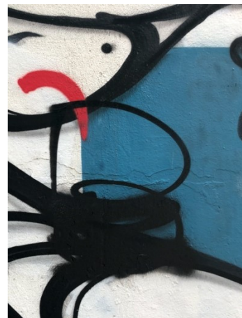
Fig. Att. 71 – Detail of vandalism with black aerosol paint over the various chromatic layers.
