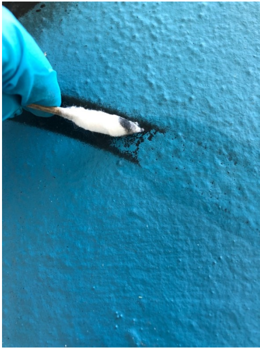
Fig. Att. 86 – Chemical cleaning in blue colour.
