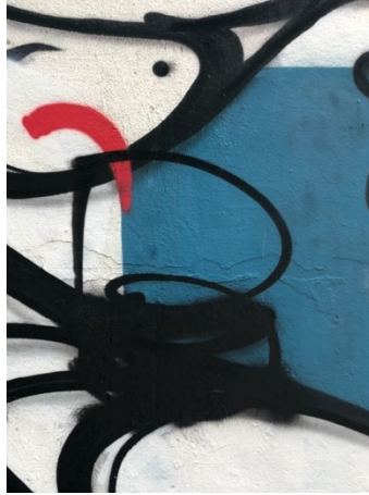
Fig. Att. 73 – Detail of vandalism with black aerosol paint over the various chromatic layers.
