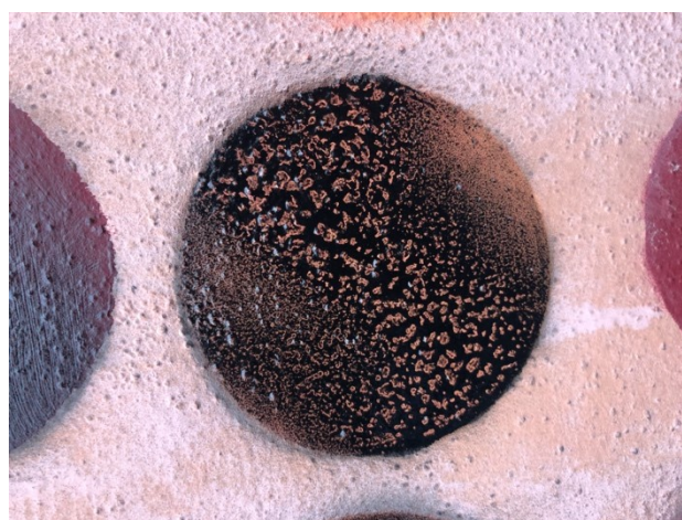
Figure 22 – Second layer of Pro-Art protective coating with vandalism.
