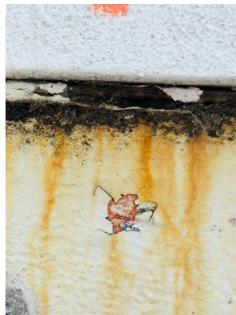
Fig. Att. 70 – Detail of the oxidation run-off on the chromatic layer.
