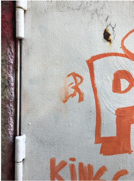
Fig. Att. 90 – Chemical cleaning in chemical cleaning of the orange marker on the water meter compartment cover.
