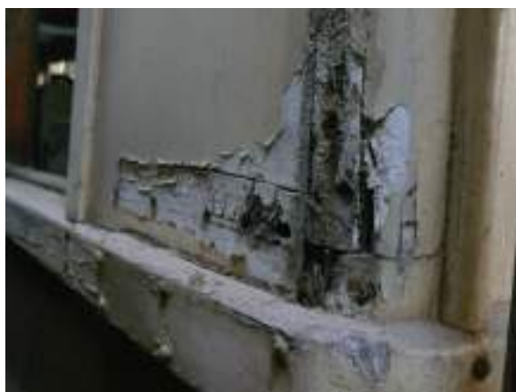
Fig. 8 - A gap on the wooden support which must be consolidated.
