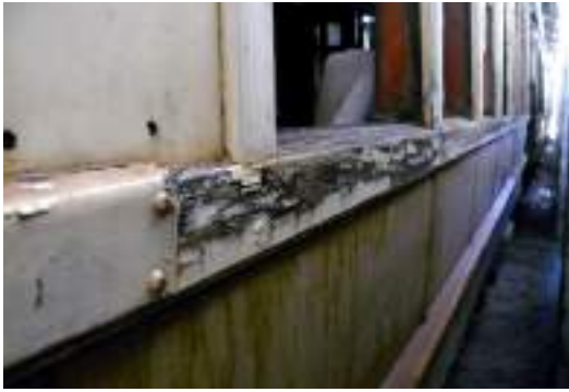
Fig. 3 - Loss of tram side paint and primer layer.
