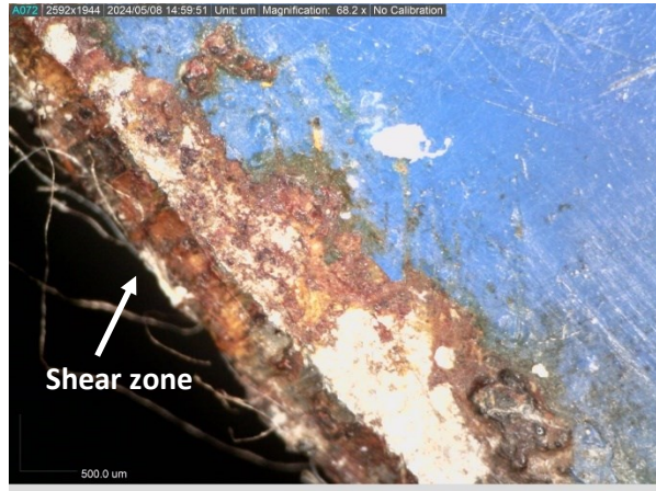
Figure 62. Shear zone under a digital microscope. Corrosion can be seen along the cut.
