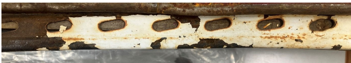
Figure 64. Loss of adhesion, and discoloration of the coating due to the corrosion of the metal substrate in Mabunda's sculptures.
