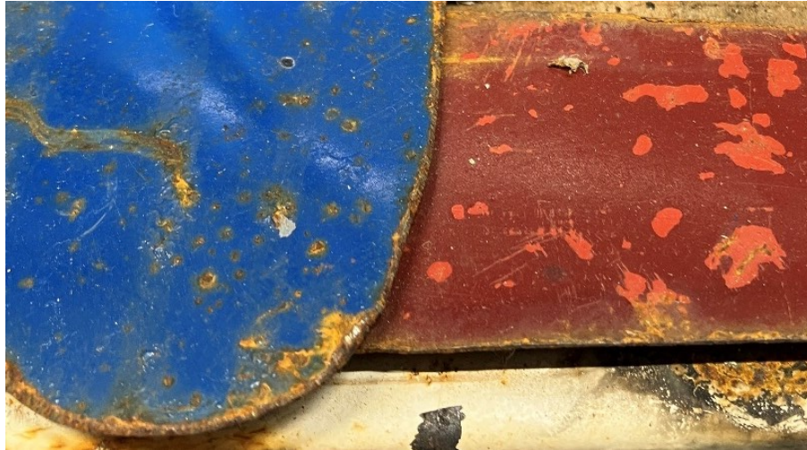
Figure 60. The formation of corrosion in the locations where the blue coatings were damaged can be seen. Meanwhile, the red coated metal shows that the existence of an intermediate layer protected the metal substrate where the topmost red coat have disappeared.
